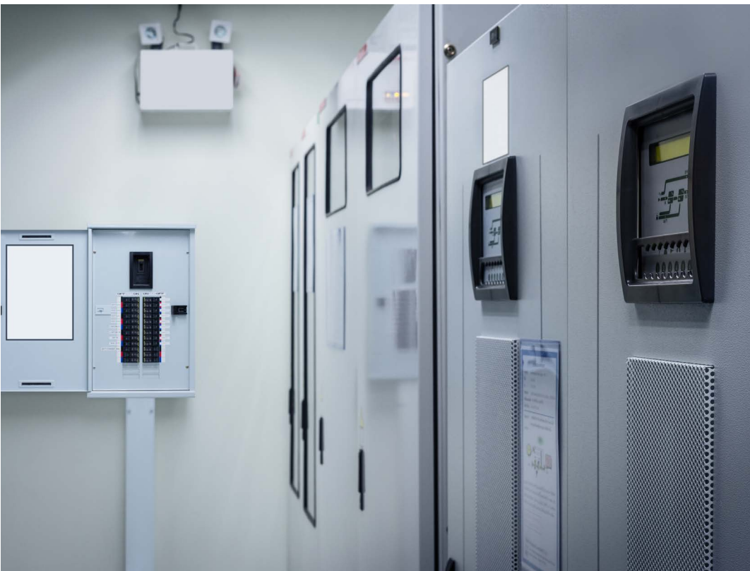
Uninterruptible Power Supplies (UPS)
